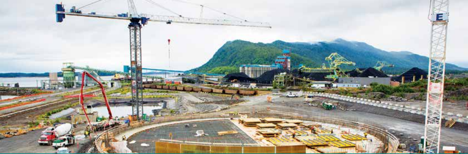
Propane tank foundation.
