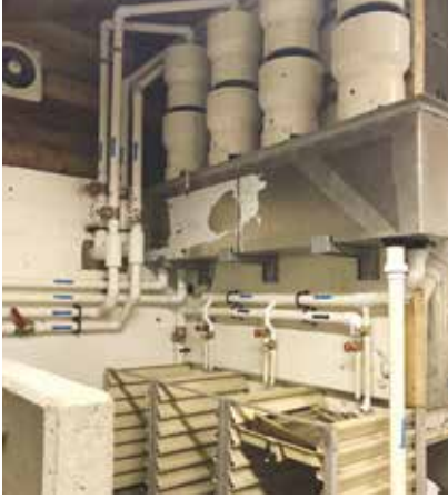
New equipment includes industrial-grade chillers and pumps, as well as improved water capacity.
